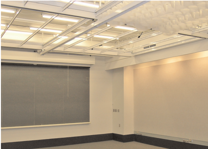
An innovative ceiling grid provides on-demand virtual rewiring for equipment and lighting.
